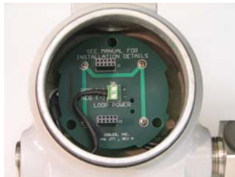
Photograph No. 2 Termination Board
